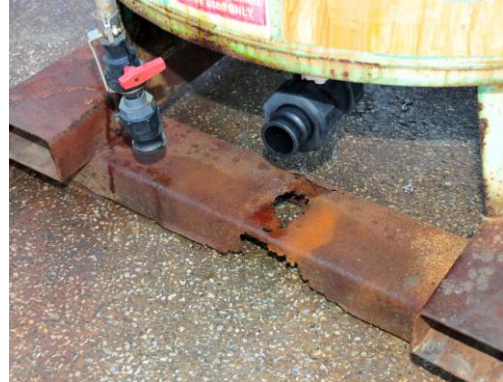
Typical corrosion of a PCM pallet base
